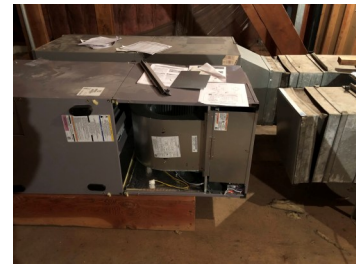
Moline Dining Hall HVAC systems in attic.
