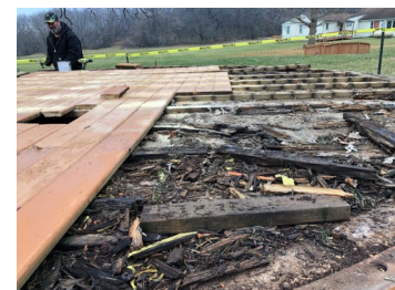
Rotted boards at Drama Drum
